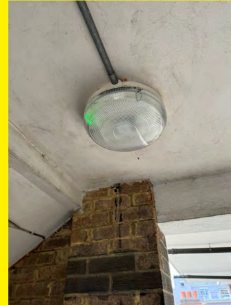
Emergency lighting at Tresham House.
