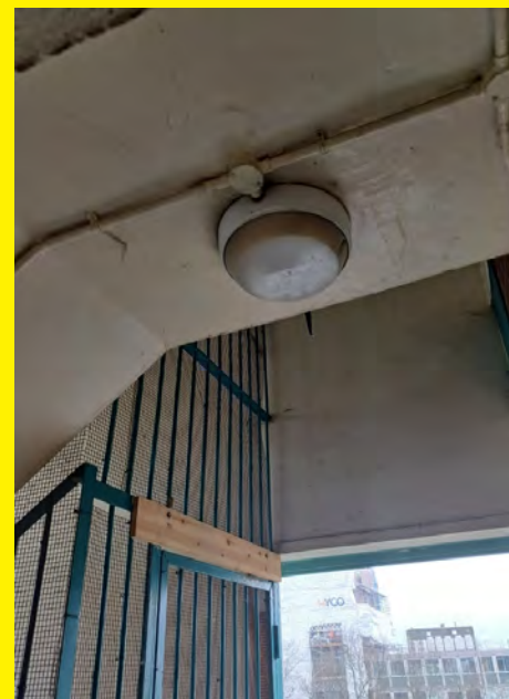
Emergency lighting at 1-19 Peperfield.
