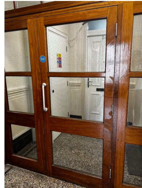
Communal Fire Door at 1-23 Trentishoe Mansions.
