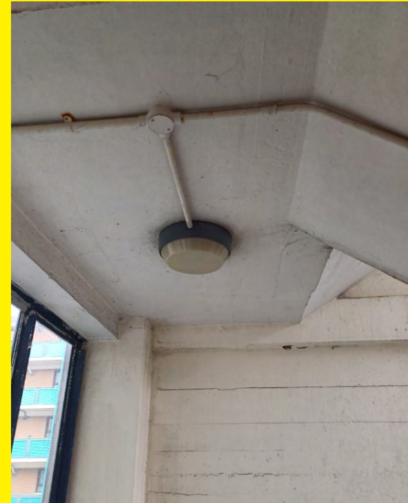
Emergency lighting at 1-24 Great Croft.
