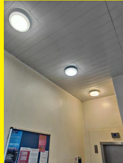
Emergency lighting at Fleetway.
