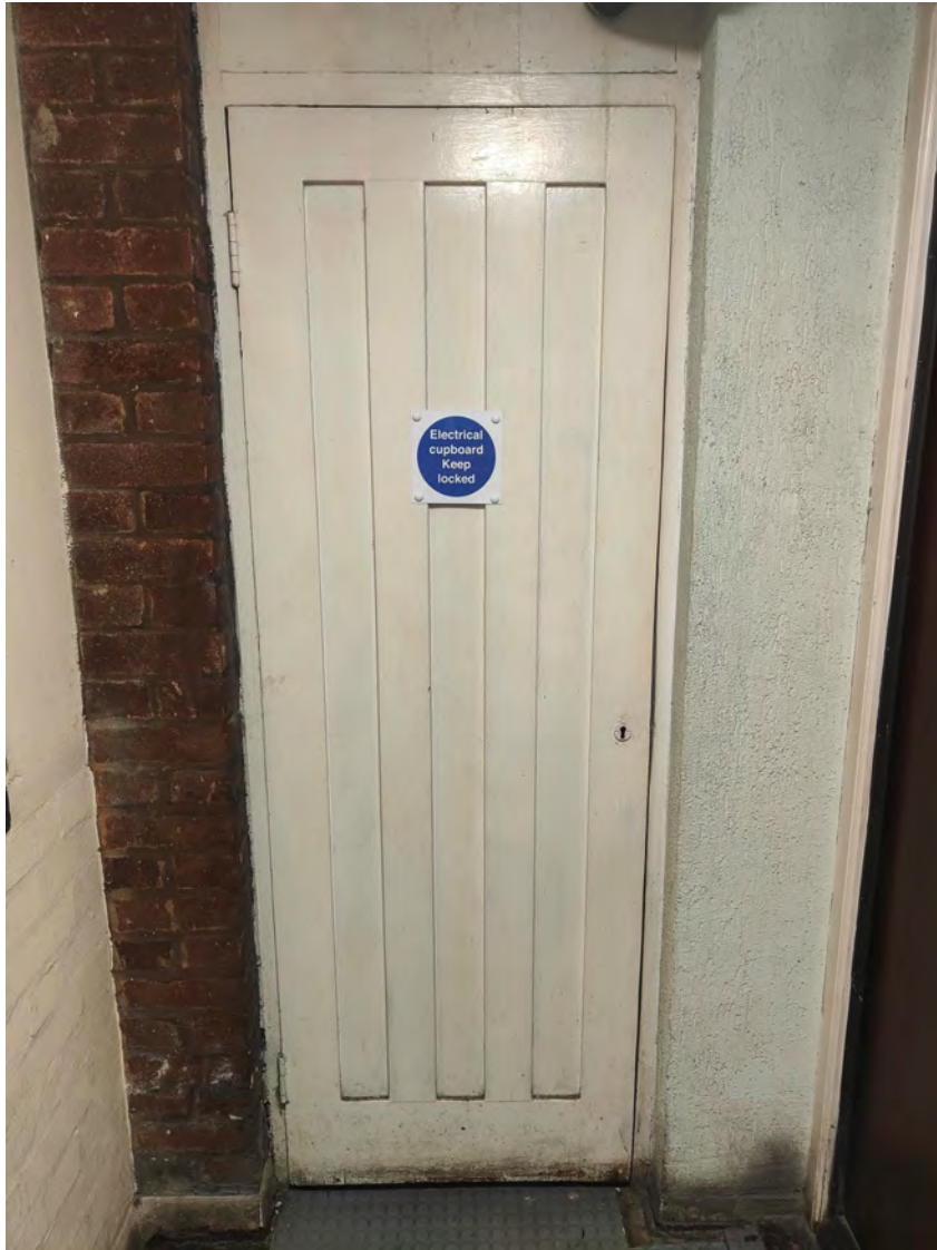
Electrical intake cupboard fire door at 1-25 Fleetway.
