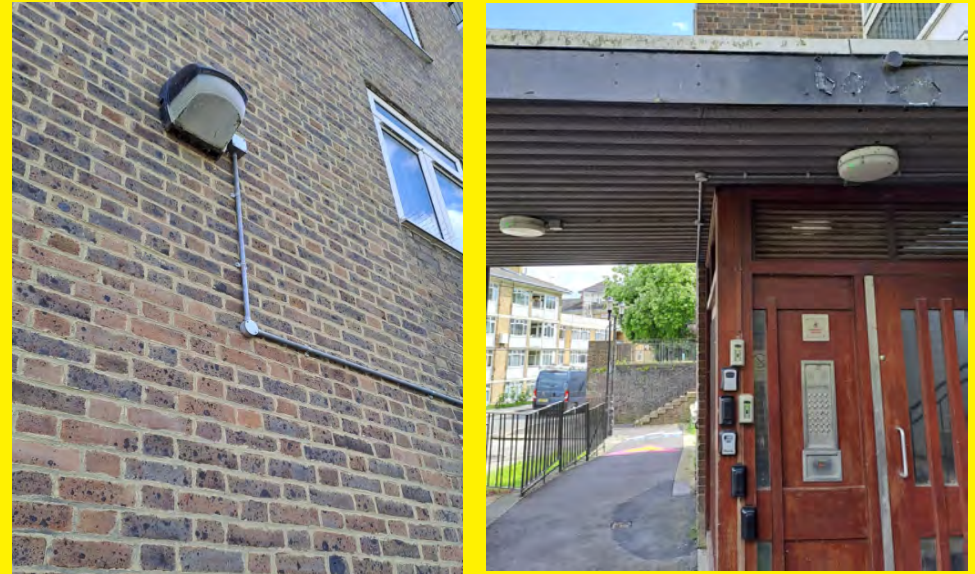
Emergency lighting at 1-27 Hazel House.
