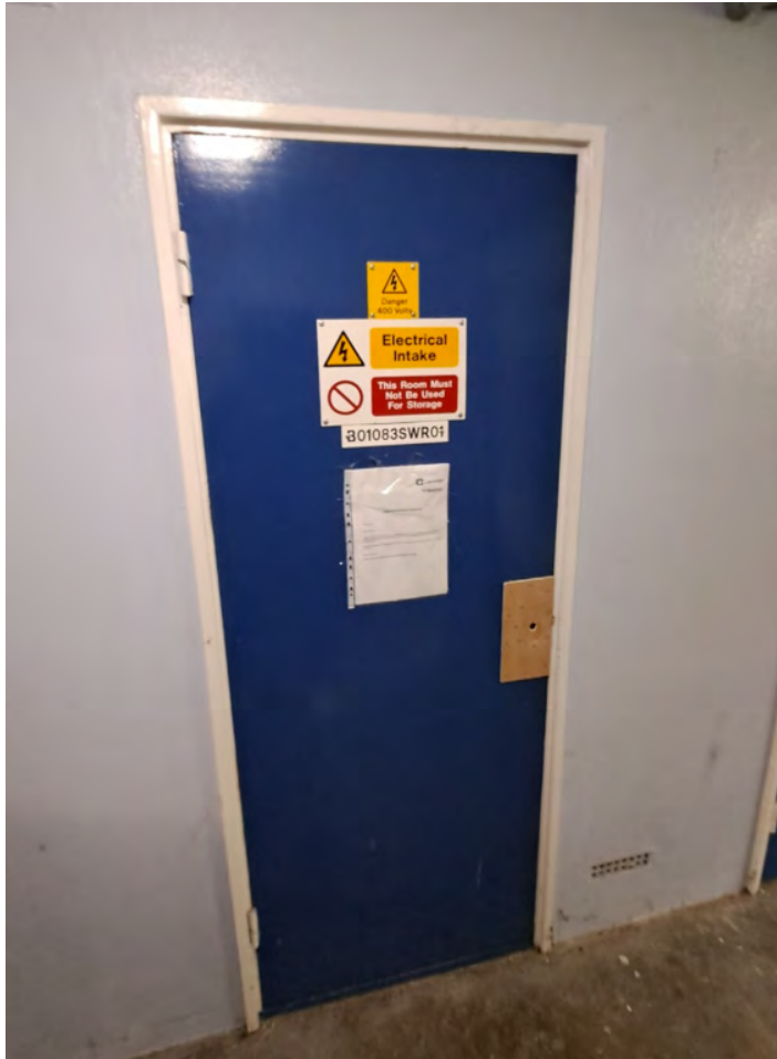
Electrical Intake Cupboard Fire Door at 1-27 Hazel House.
