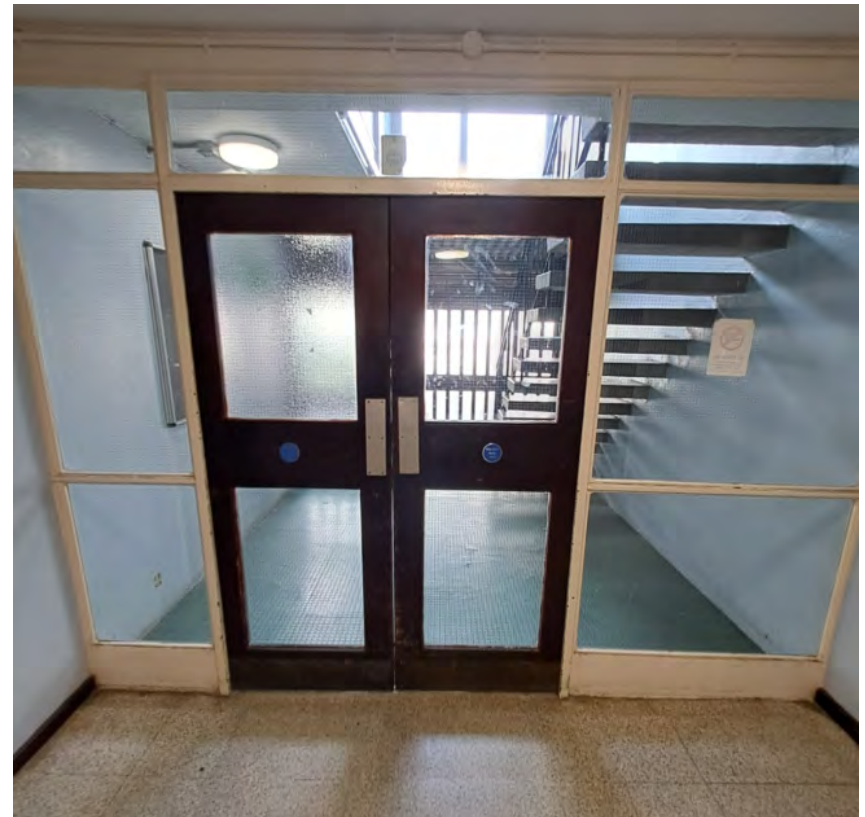
Communal Fire Doors at 1-27 Hazel House .
