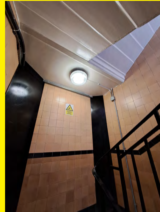
Emergency lighting at 1-32 Mead Close .
