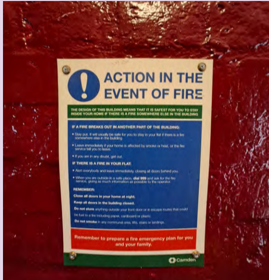
Fire Action Notice at 1-32 Mead Close .
