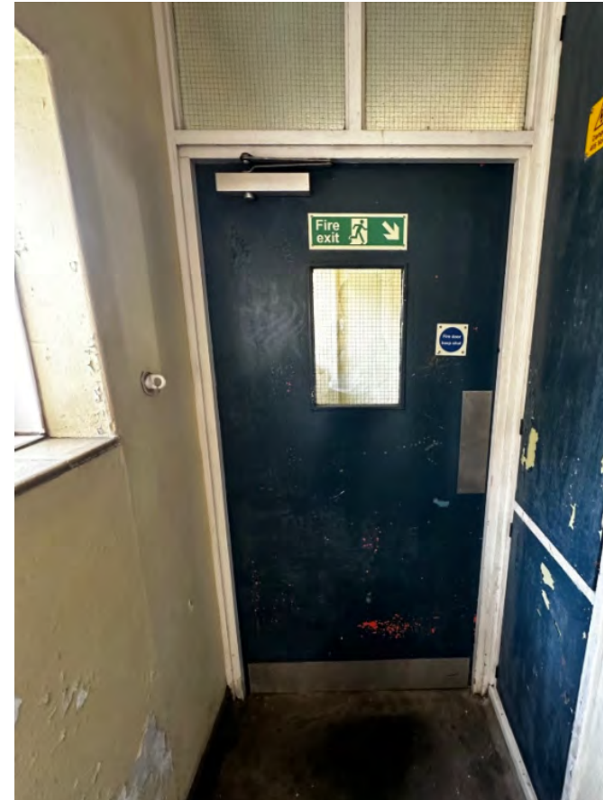
Communal Fire Door at 1-33 Mullen Tower.
