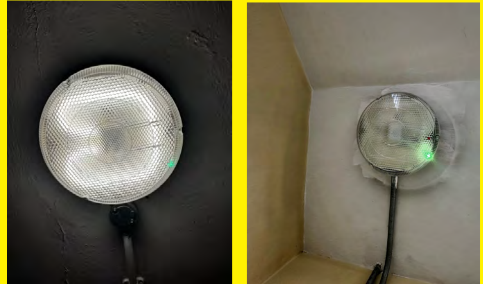
Emergency lighting at 1-33 Mullen Tower.
