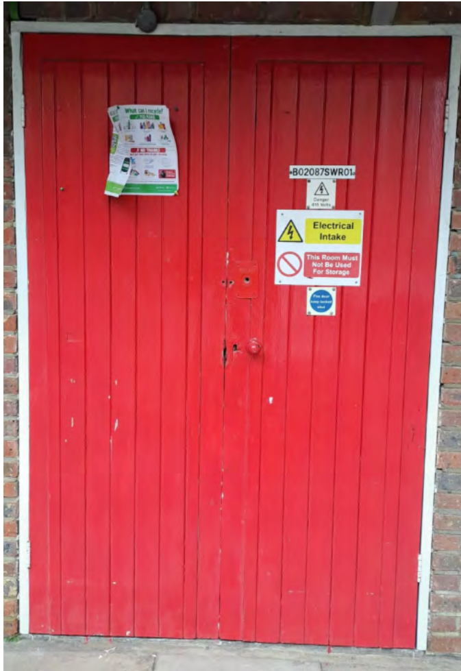
Electrical intake cupboard fire door at 1-43 Hickes House.
