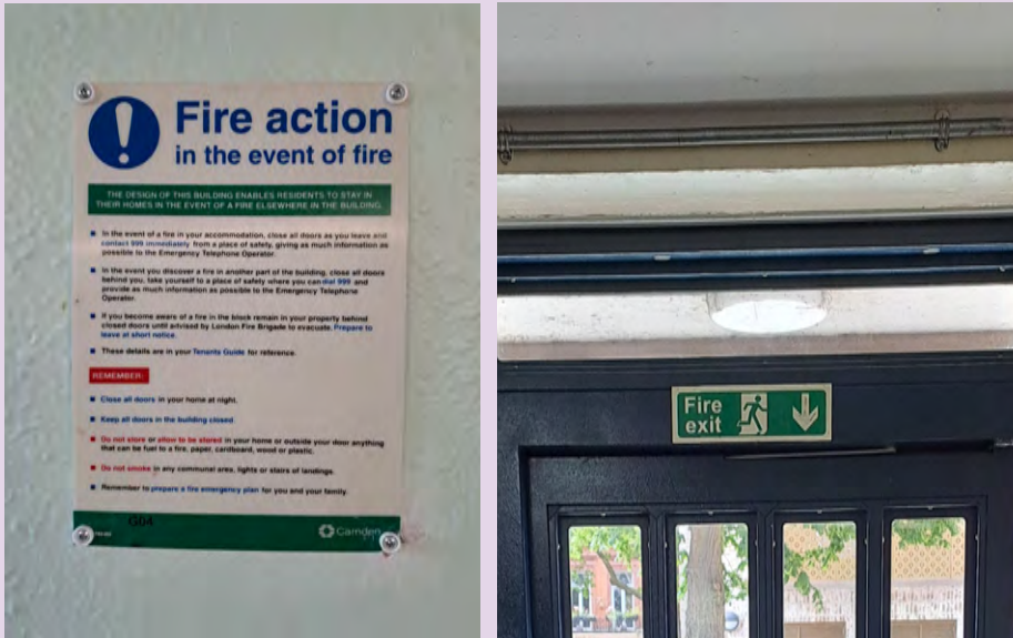
Fire Action Notice and Fire Exit Sign at 1-44 Swallowfield.
