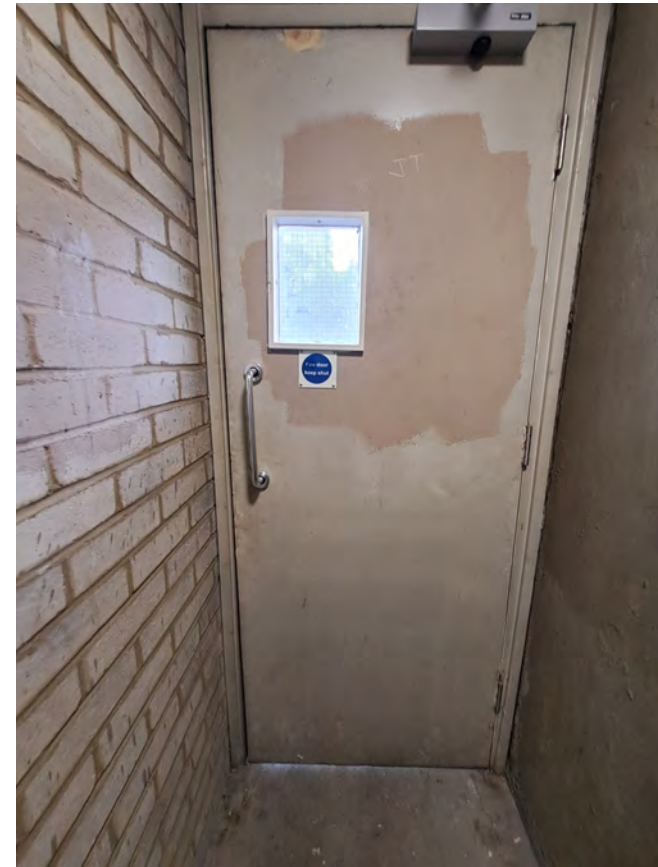
Communal Fire Door at 1-44 Swallowfield.
