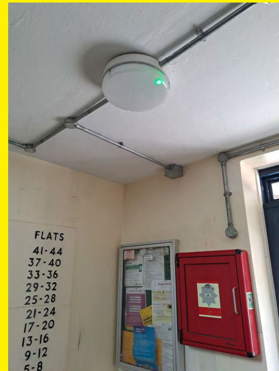
Emergency lighting and Secure Information Box at 1-44 Swallowfield.
