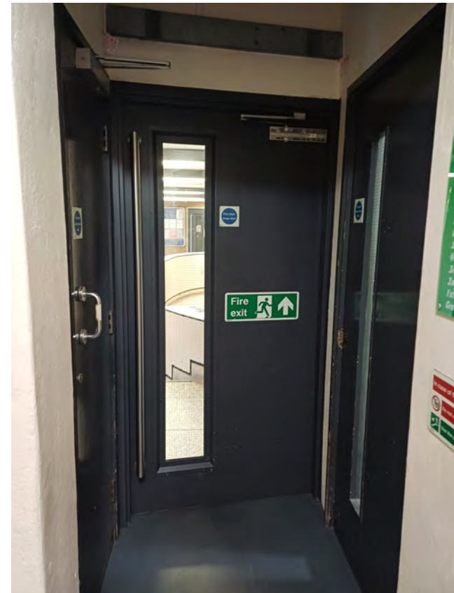
Communal Fire Door at 1-48 Glynde Reach.
