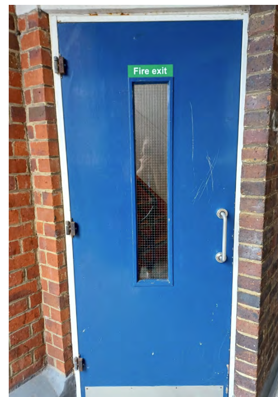
Communal Fire Door at 1-56 Torbay Court.
