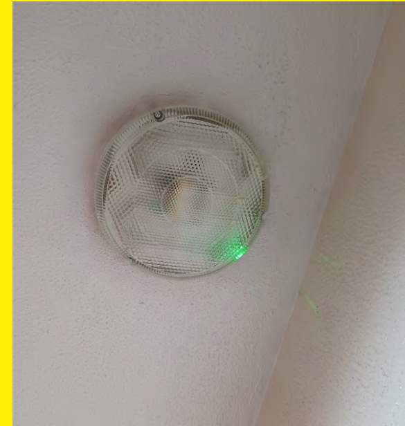
Emergency lighting at 1-56 Torbay Court.
