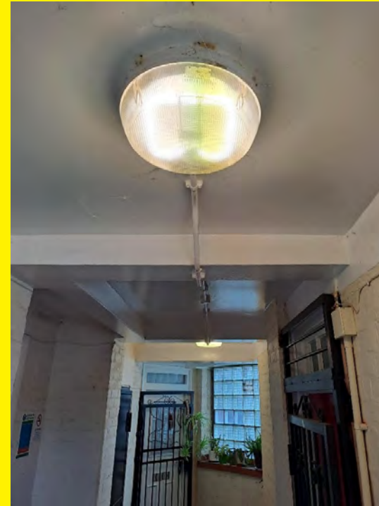
Emergency lighting at Greatfield House.
