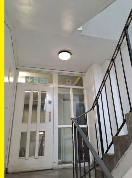
Emergency lighting at Burmarsh.
