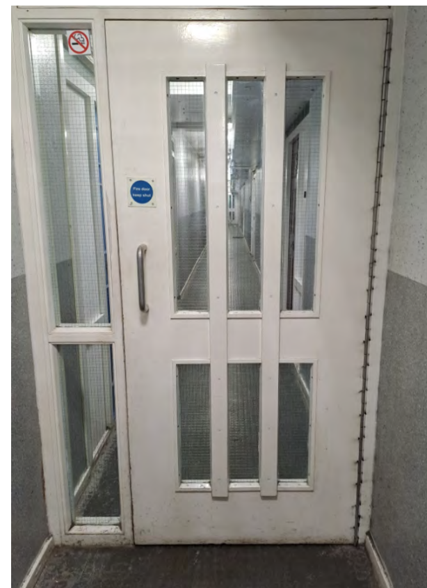
Communal Fire Door at Burmarsh.
