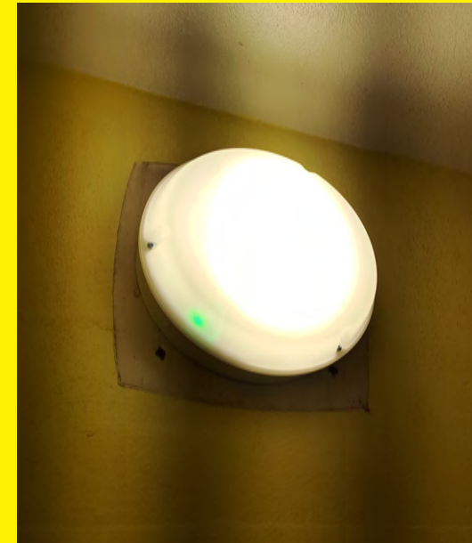
Emergency lighting at Dalehead.
