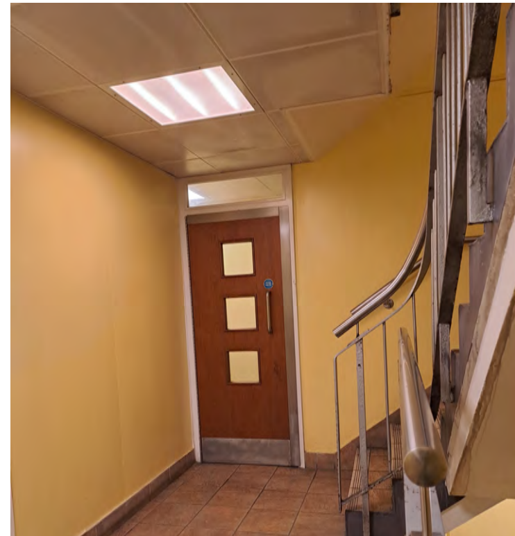
Communal area fire door at Dalehead.
