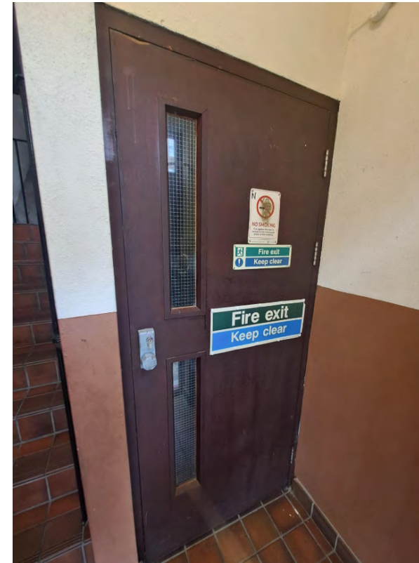
Communal Fire Door at 2-42 Laney House.
