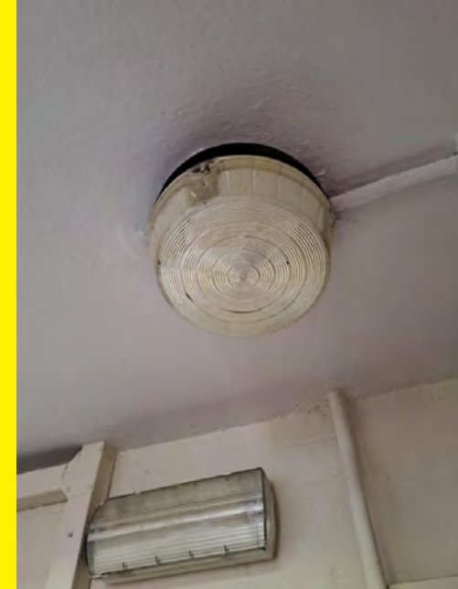
Emergency lighting at 2-42 Laney House.
