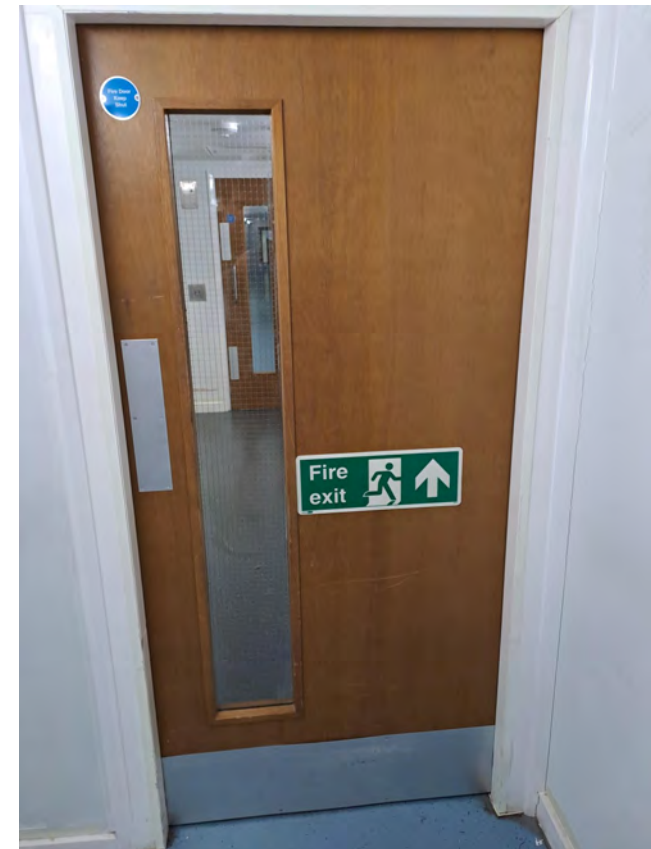
Communal Fire Door at Grafton Way.
