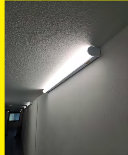
Emergency lighting at Grafton Way
